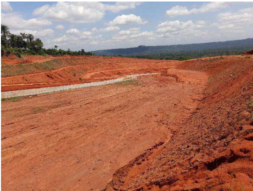
Section view of Urualla erosion site
